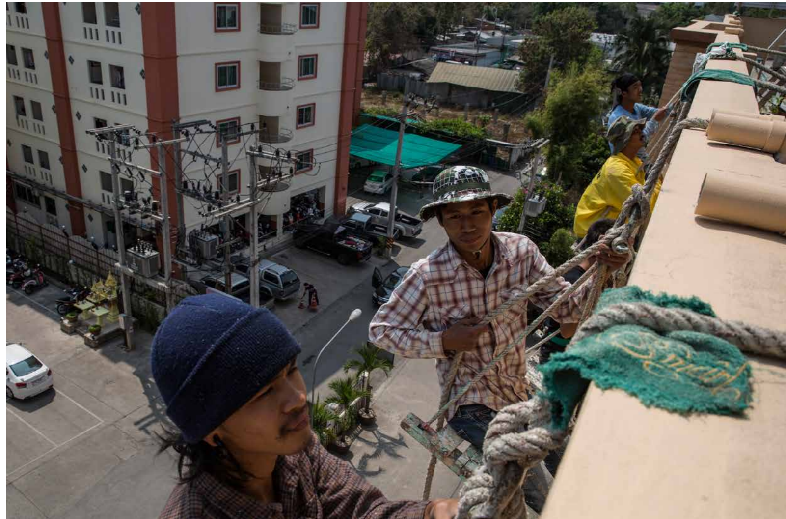
Workers painting building in Chiang Kian, Chiang Mai. Photograph by Matthew Sherwood.
